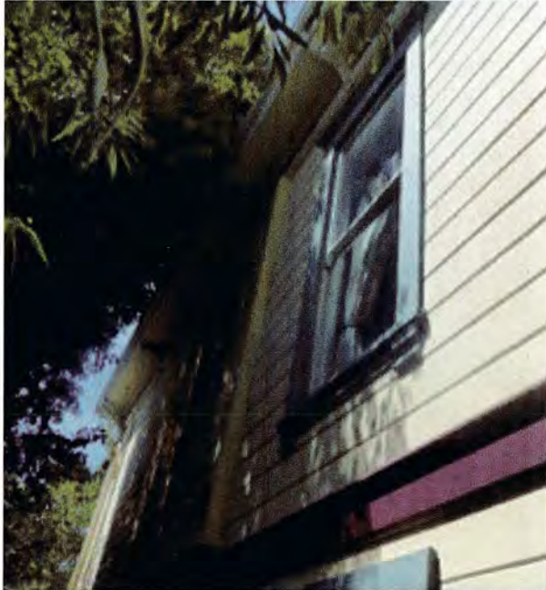
Figure 8: Left. East facade detail, showing double hung window with exterior casework, horizontal board siding, water table between basement level and main floor, and boxed eaves. Photo 2019.
